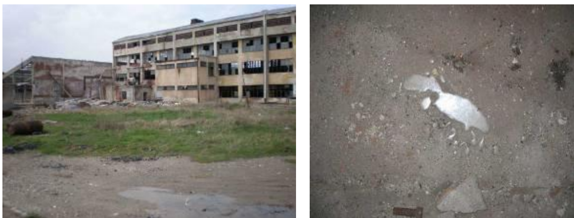
Figure 18. Former electrolysis plant (view from NE towards SW) (left) and former electrolysis plant – inside, massive Hg spillage (right)
